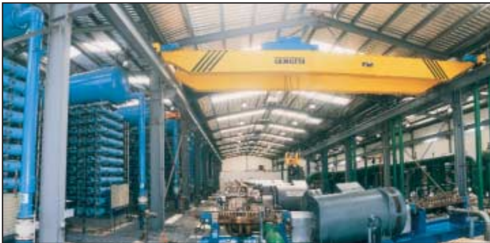
Dhekelia Desalination Plant
