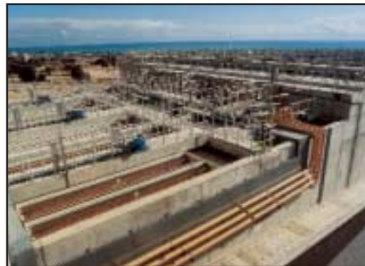
Limassol Water Treatment Plant
